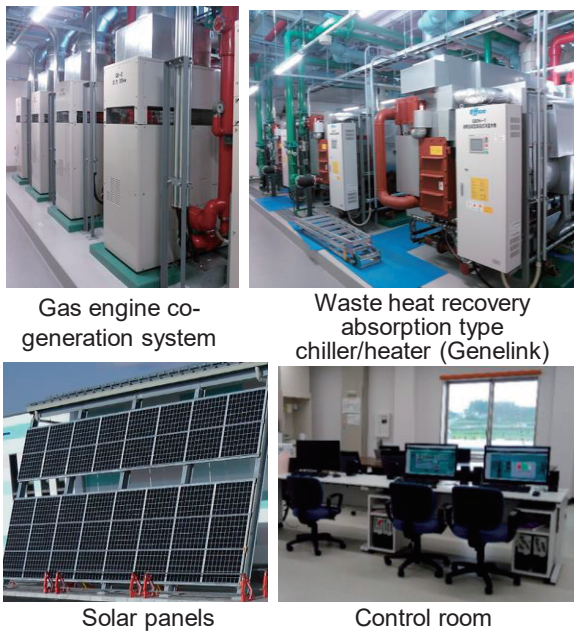
Fig. 6 Main equipment at the Shinchi Energy Center.
