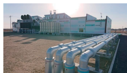
Heat supply conduits on the north side of the building
