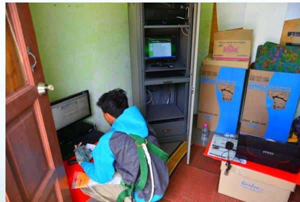
Checking od captured data at Gateway
